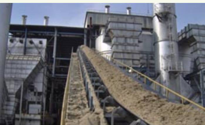
Renewable electricity generation • Verified by DNV ( www.dnv.com ) Annual GHG reductions (whole project): 79,400 tonnes CO 2 e
